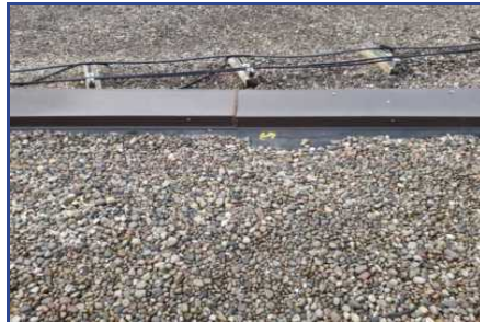
Section A - Deficiency #1 deficiency photo before
