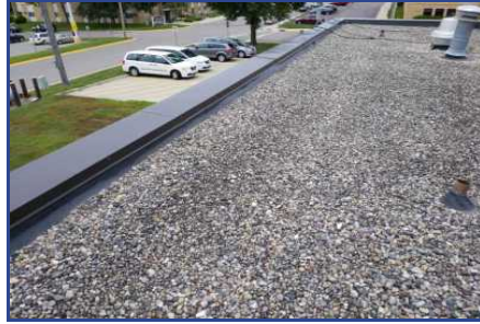
Section A - Deficiency #1 Membrane shrinkage at walls
