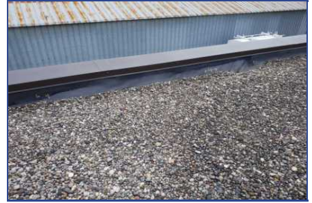
Section A - Deficiency #1 Membrane shrinkage at walls
