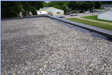
Section A - Deficiency #1 Membrane shrinkage at walls
