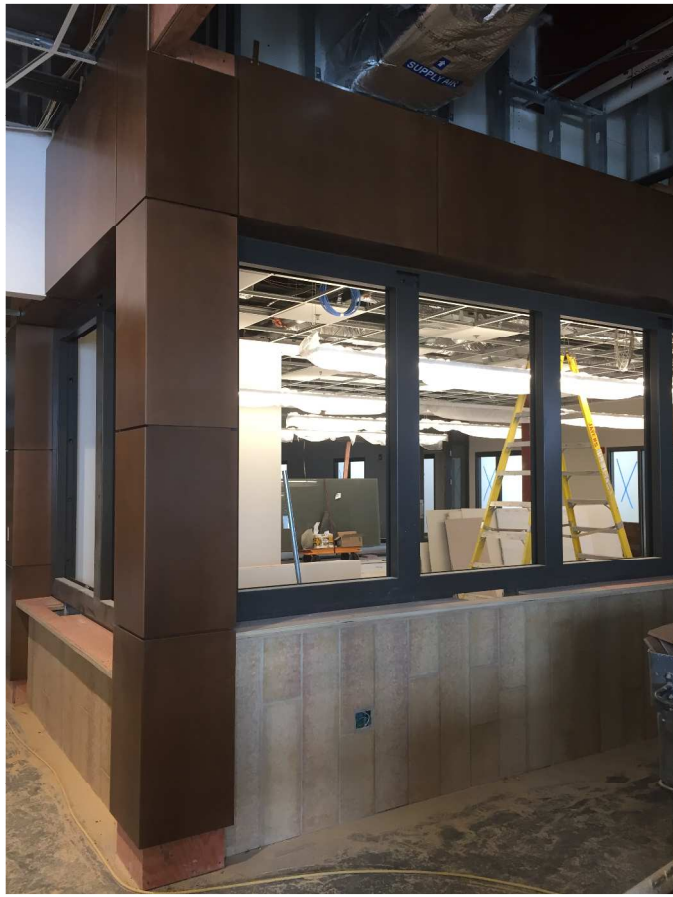
Wood paneling started at the Sheriff Administration desk this week, wrapping the Vetter stone accent!
