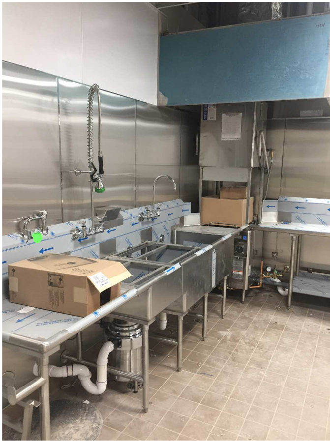
Kitchen equipment was delivered and began install this week. This includes sinks, counters, shelving and cooking equipment!
