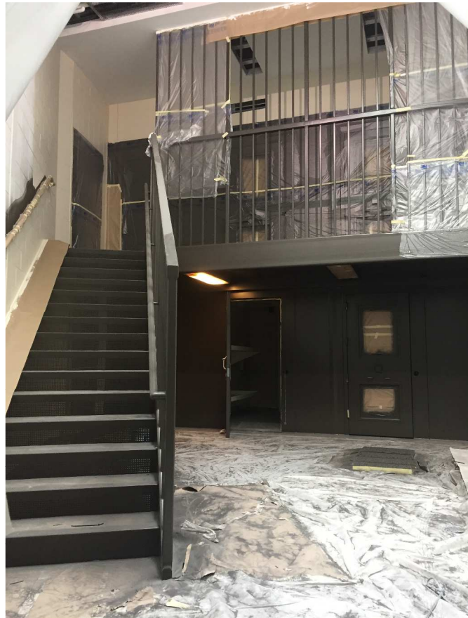
Painting activities continued throughout the day rooms in the jail. Painting the steel, cells and walls!
