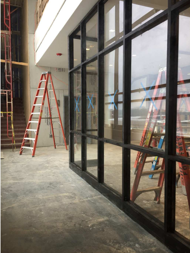
The last few panels of interior storefront at the main lobby were installed with glass! Making way for the finishes in this area!
