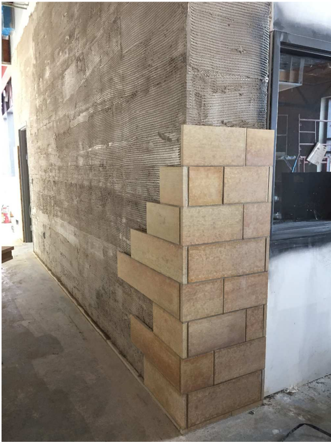
The last wall of interior stone on the second floor began with detailing the corners and base!
