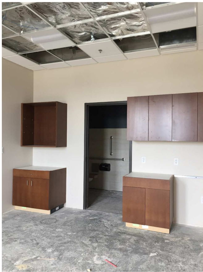
Upper and lower cabinets were set in the judges chambers on second floor!
