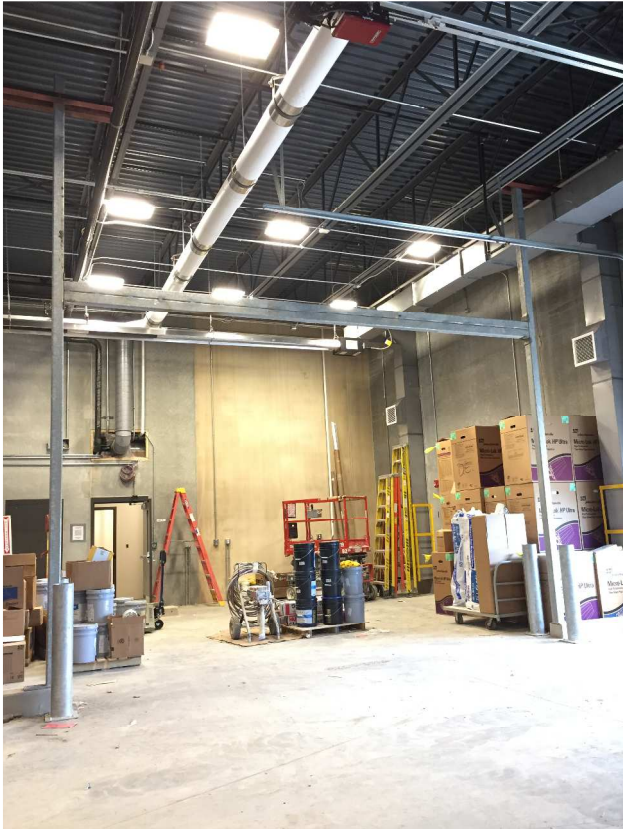
The steel was installed and welded for the vehicle processing overhead door!
