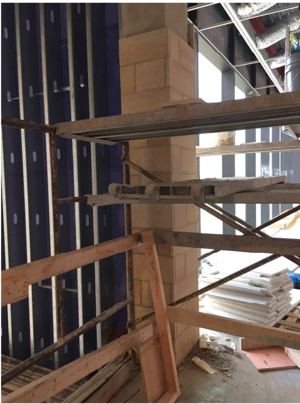
The remaining interior stone on the second floor is being installed on interior columns!
