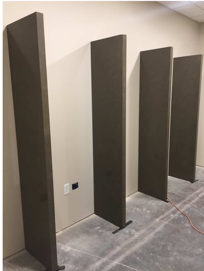
Quartz dividing walls installed in video visitation for privacy on the kiosks
