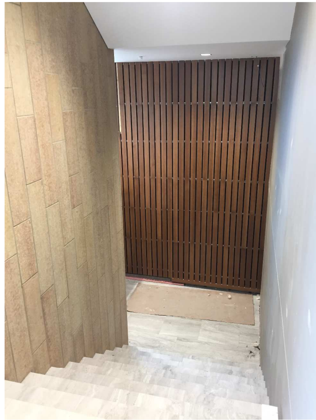
Wood decorative wall is going up in the main stairwell around the lobby elevator!
