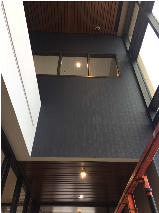
Wall covering started as well as the continuation of wood ceilings installed in the main lobby opening!
