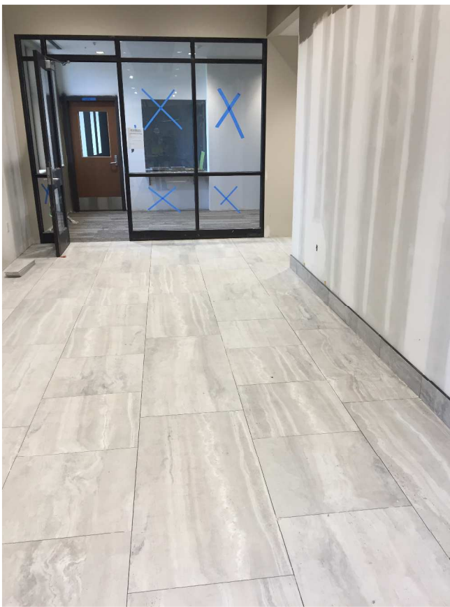
Floor tile and base was installed in the main lobby and corridor! Grouting next week
