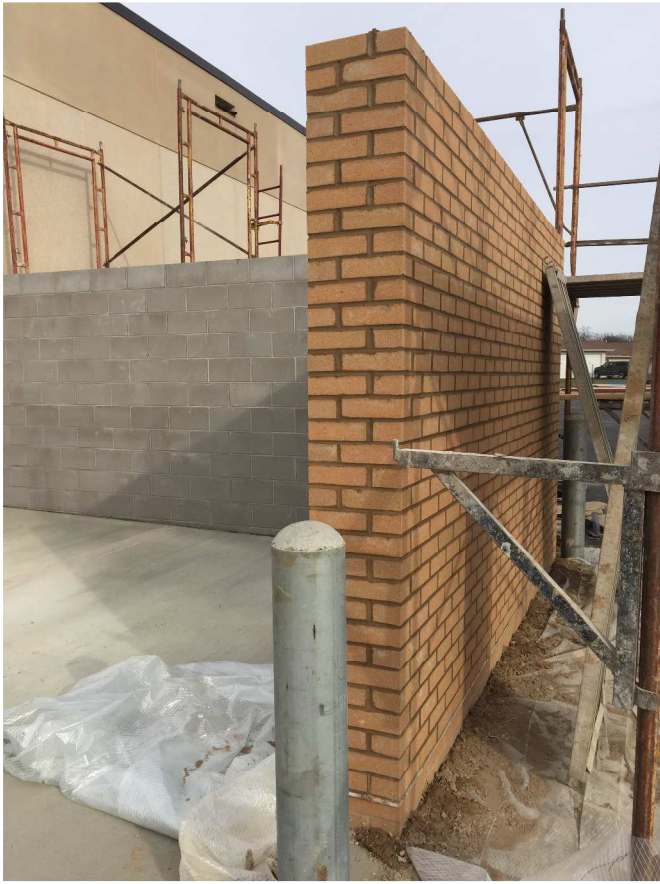
The trash enclosure masonry walls received a layer of brick to match the building. Steel bollards were installed and finished with concrete as well bringing the trash enclosure one step closer to completion!
