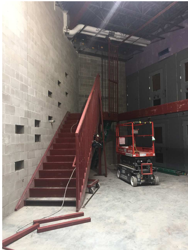
The day room steel work has begun. This include steel beams for the mezzanine levels, stairs and guardrails that will install along the mezzanine level!
