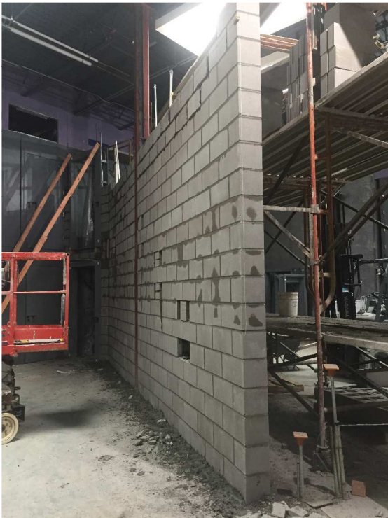
Masonry walls continue in the jail area as well as rough ins in the newly drywalled walls above the cells!
