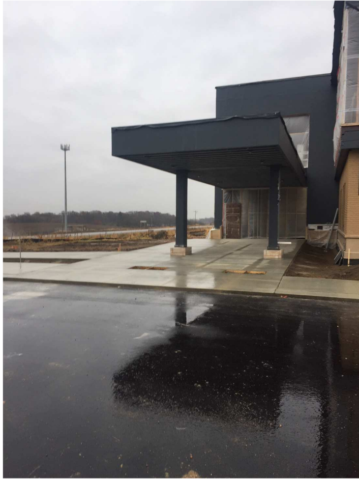
The main entrance was poured and saw cut late this week, covering the newly installed snowmelt system and creating a finished product! The openings are for the exterior benches
