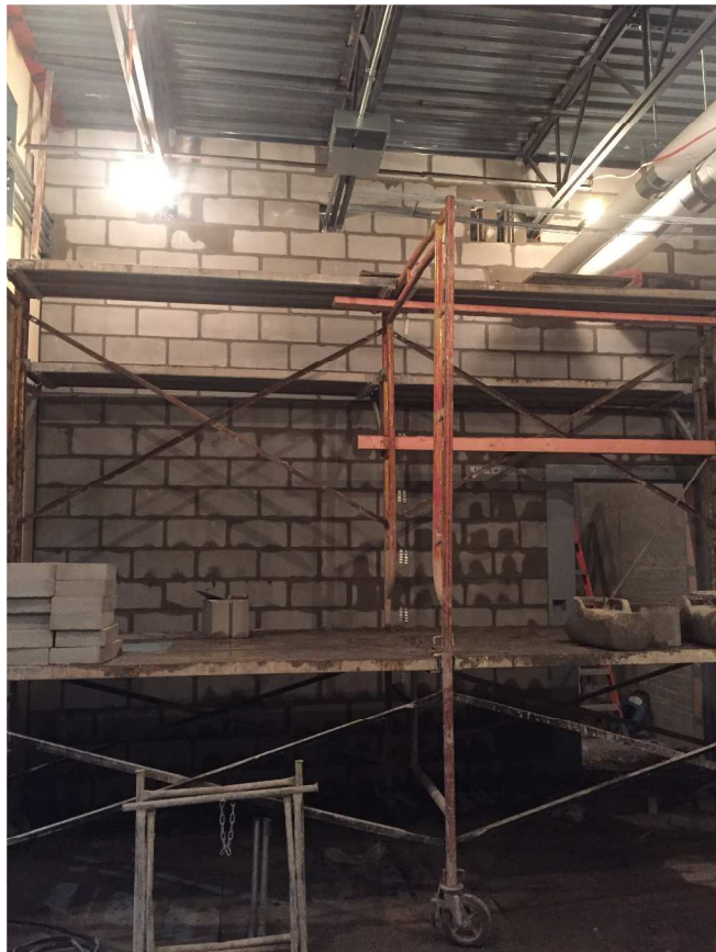
The last few walls in the Jail and Work Release areas are completed, leaving only Master Control left for masonry!
