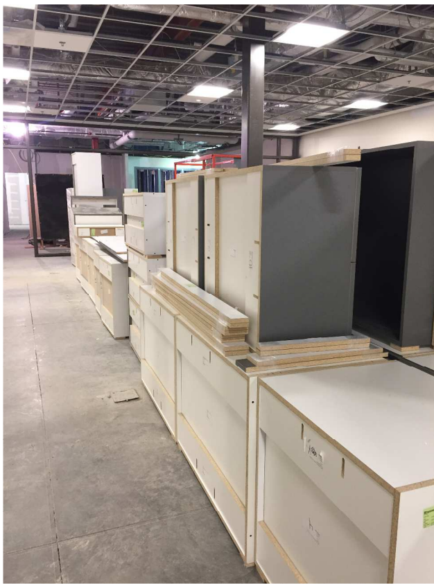
First floor casework has been delivered, acclimating to the temperature and humidity of the building making them ready for install next week!
