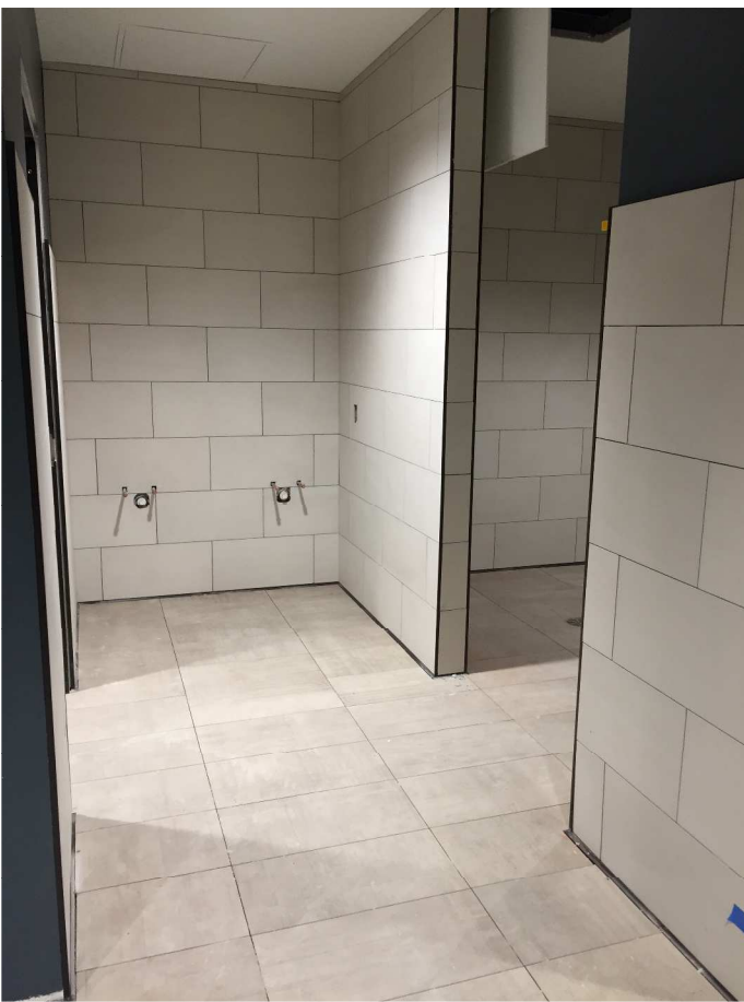
The lower level locker rooms were fully tiled, floor and wall. They will receive grout next week!
