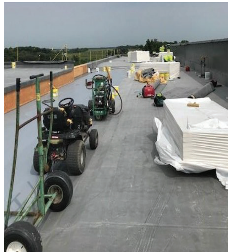
Roofing on Area A is progressing nicely. This area should be completed by Monday or Tuesday of next week.
