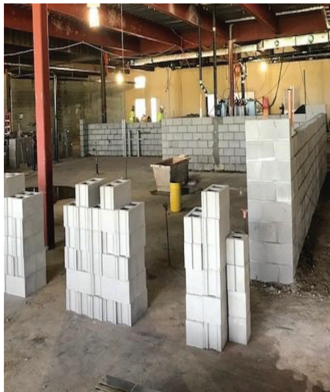
The masonry crew began laying their CMU walls in Area A. These walls will be for the dispatch and sallyport rooms.
