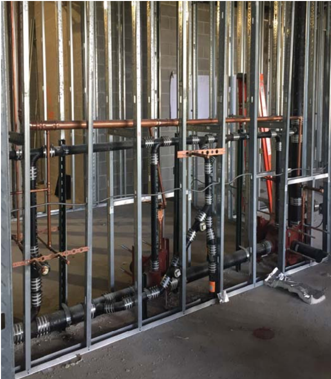
In wall MEP rough ins have started on the lower and main levels.
