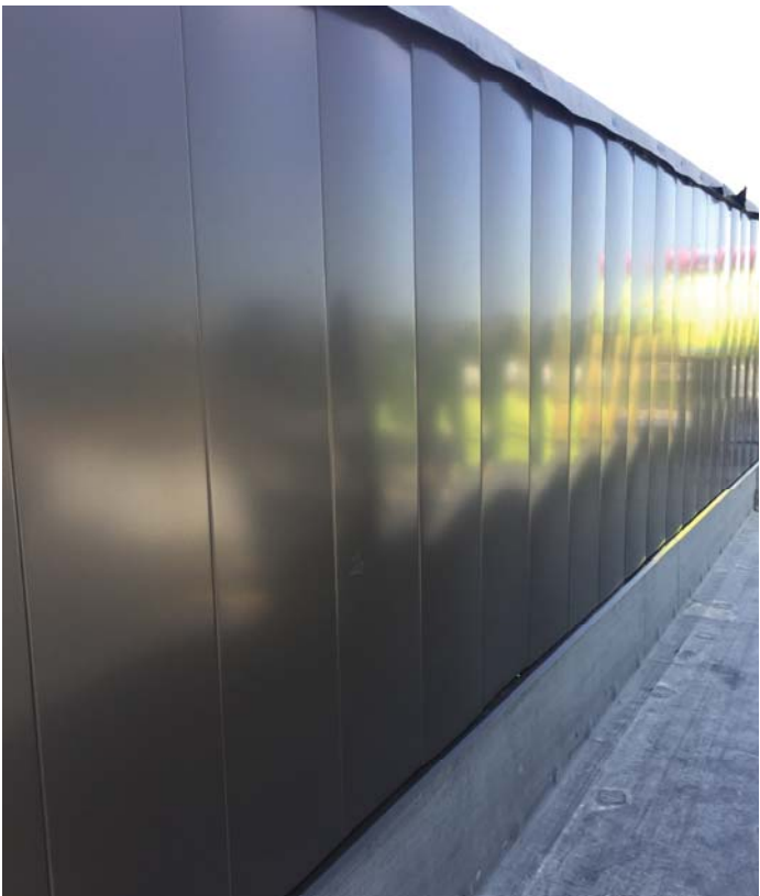
Metal Wall Panels have begun being set on the exterior of the building.
