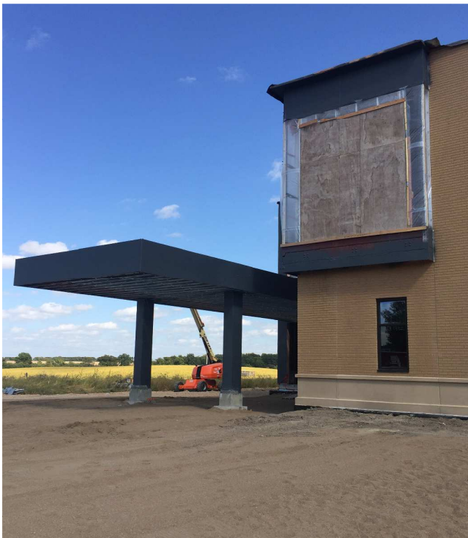
Air barrier was sprayed on the entry way canopy. Also, another opening was temporarily enclosed.
